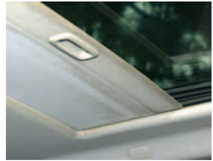
Slight panel discolouration through day to day usage and wear.
